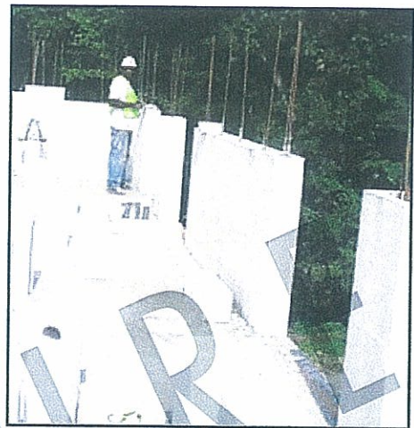
Installation of AAC reinforced block walls at State University of New York at Stony Brook.
